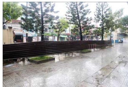
Figure 1. Typhoon caused wall collapsed in Phan Dang Luu PS in 2018 (Source: Vietnam News Agency)
